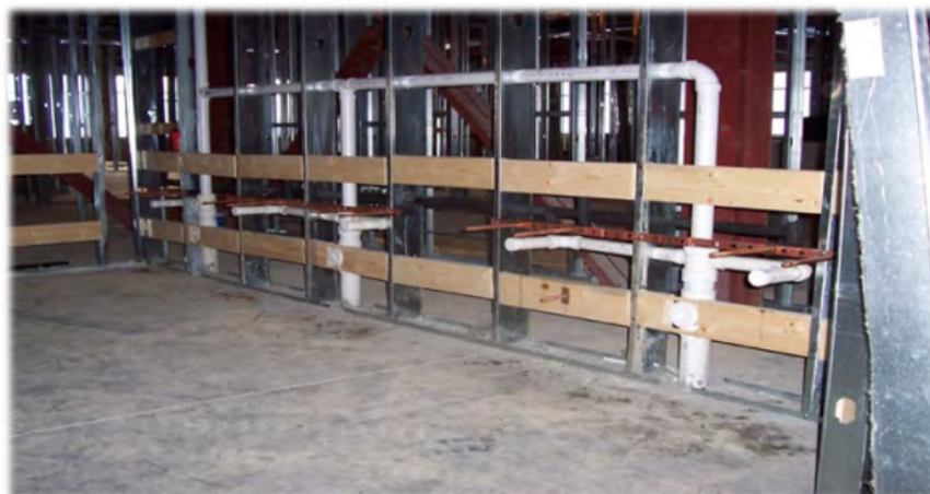
Photo of a typical multiple lavatory rough-in
